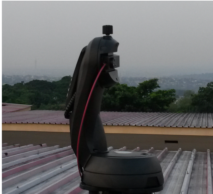
Figure 3.1: Motorized mount for version 1 of the MAX-DOAS instrument installed on the roof of Faculty of Science of UniKiN.
