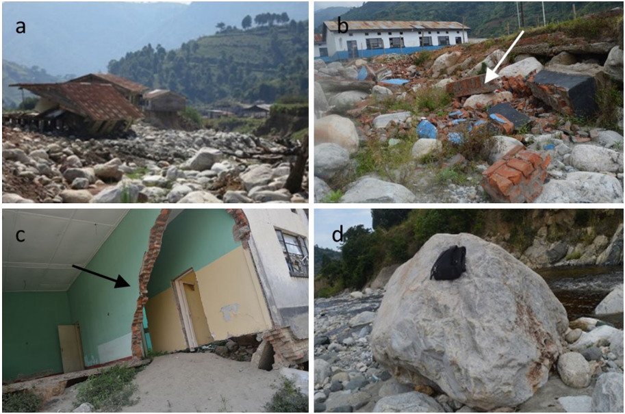
Fig. 14 Examples of damage caused by the flood. a River bed and scour, b destruction of house foundation (white arrow), c destruction of house due to impact from debris (black arrow), d illustration of boulder size frequently found in the valley (black bag on the boulder is ca. 40 cm high, location: Fig. 13a)
