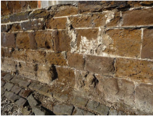
Figure 2. A typical example of damage to the ferruginous sandstone at the St. Catherine's Church of Kortrijk-Dutsel.
