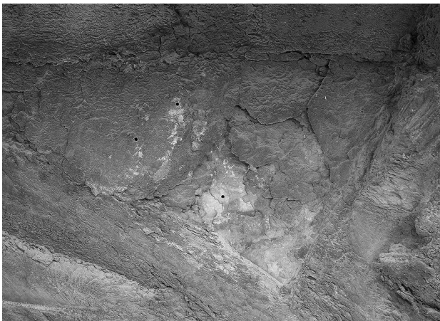
Fig. 4 Face-bedded block showing multiple delamination (Capitole portal, spandrel at the right side) © KIK-IRPA (Monuments Laboratory)
