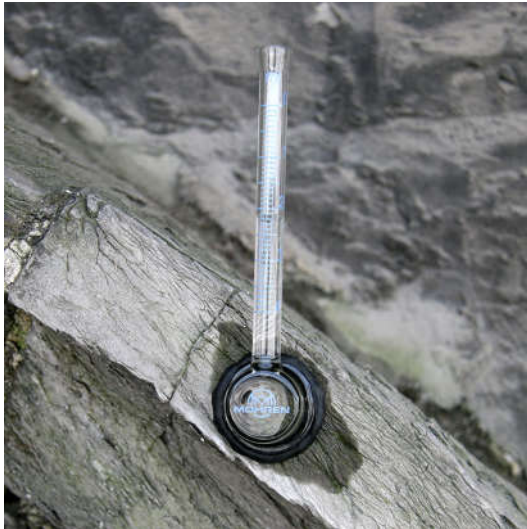
Fig. 8 Example of the formation of a wetted zone which is stretched to an ellipse shape in the direction of the bedding (dripstone of the Mantile portal) © KIK-IRPA (Monuments Laboratory)
