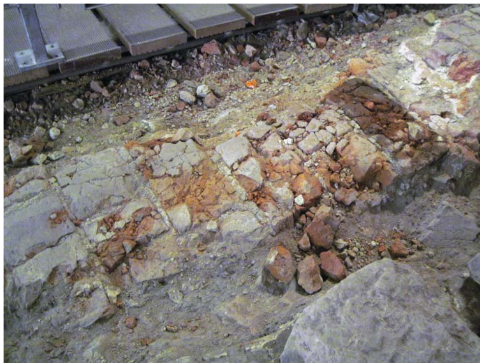
FIGURE 10 The severely fissured bricks of the Aula Magna.
