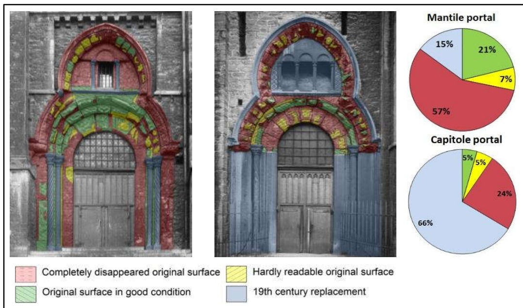
Fig. 5: General mapping and diagrams of the state of conservation of the sculpted surface. Mantile portal (left) and Capitoile portal (right) © KIK-IRPA, Brussels.
