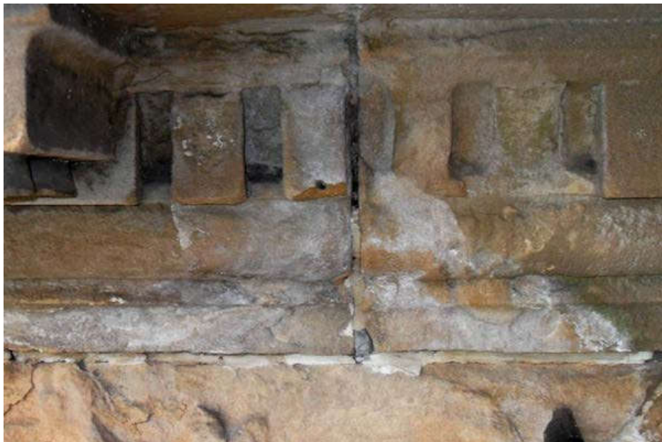
Figure 5. Zone below the cornice showing extensive efflorescence of gypsum and loss of some dentils. The outer cm of the stone contains gypsum (2 wt%, further decreasing with depth).
