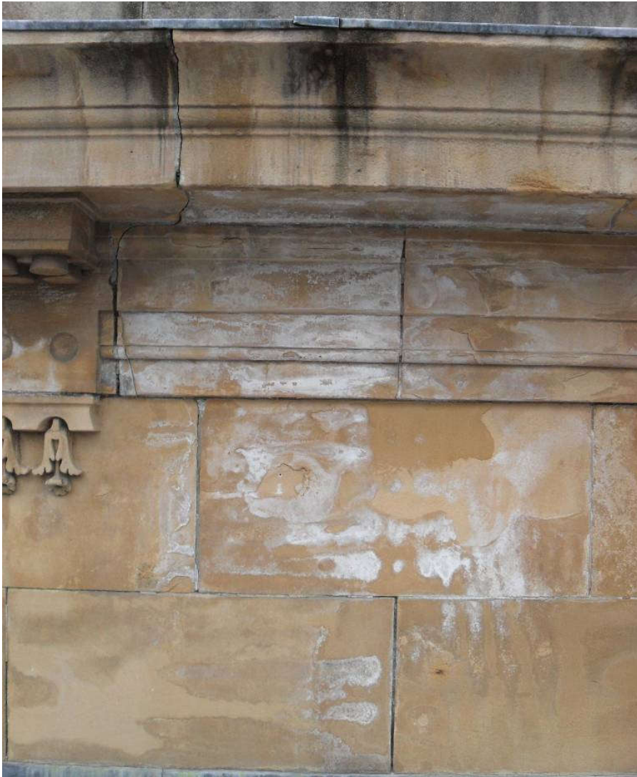
Figure 6. A high amount of gypsum efflorescence is seen, while scarce amounts of salts are detected in the underlying stone.
