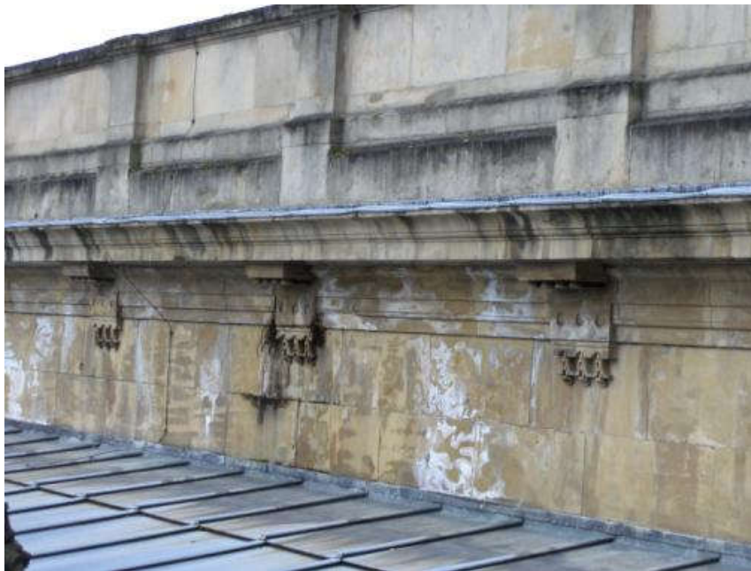
Figure 2. (Salt) staining underneath the cornice where the water evacuation system is hidden behind the wall. Two varieties of the Luxembourg sandstone can be seen: a warm yellow coloured variety below the cornice and a light grayish one above it.
