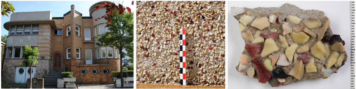
Figure 1: Façade with grey cimorné zones (De Panne, Arch. L. Legein, 1936) - detailed picture of this cimorné finish with white, beige, yellow, black and dark red glass fragments – picture of the onsite lifted sample M1 (KIK-IRPA).
