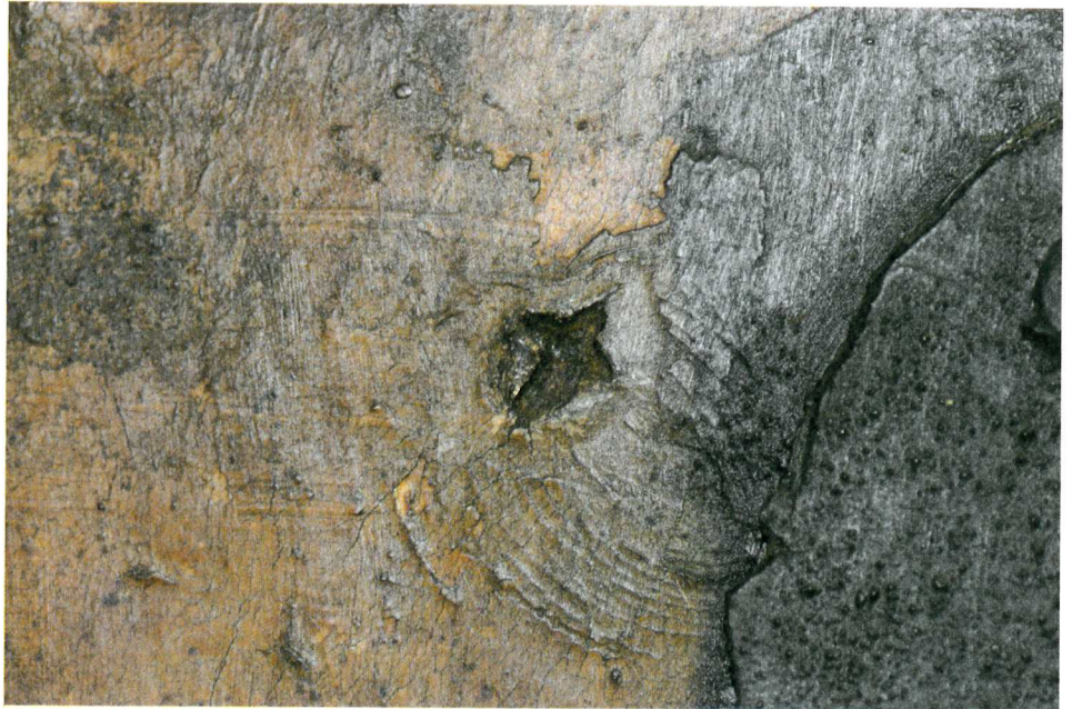
Figure 9a Cross-shaped impact damage to upper left of the grille. © C. Currie
