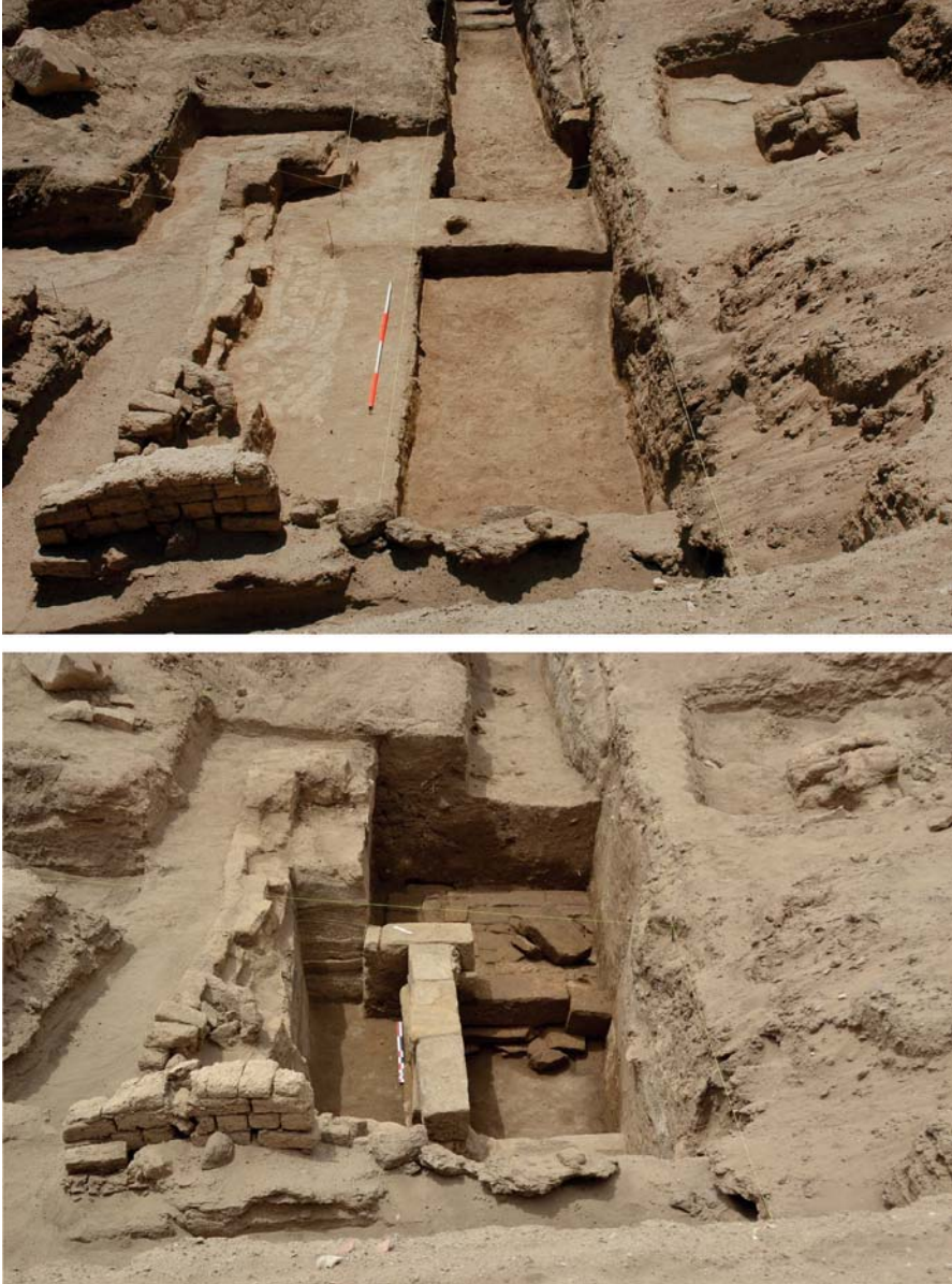
Fig. 5. Overview of the excavation before and after the discovery of the stone building. View from the north-east (© Belgian Archaeological Mission to Elkab).
